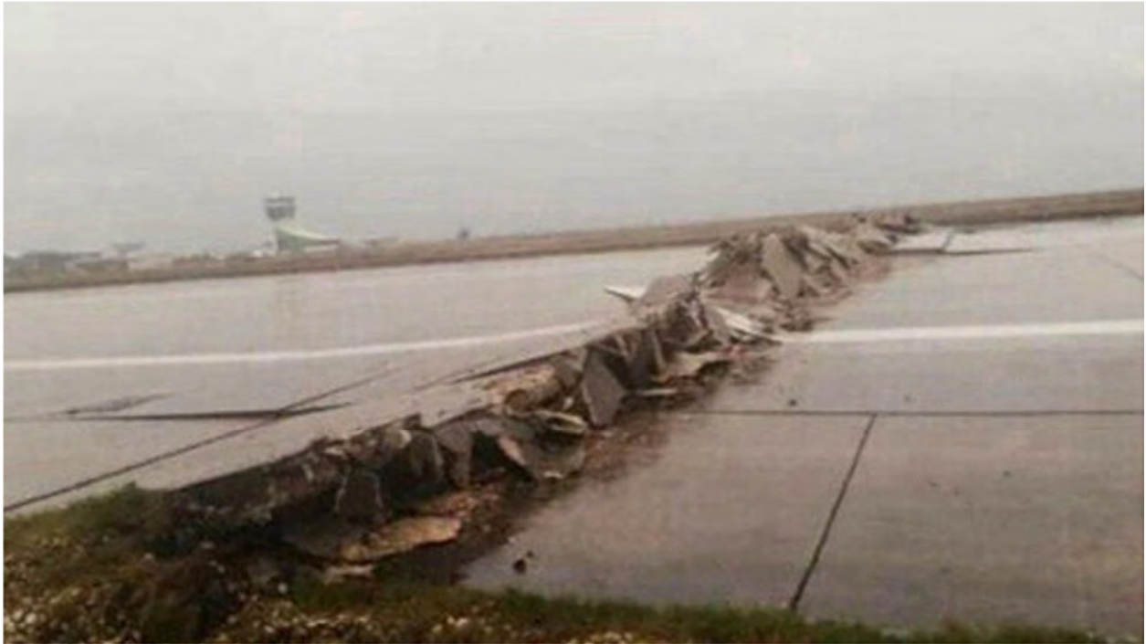
Figure 2: Damage to Hatay Airport runway ( https://www.ozgurkocaeli.com.tr/haber/13964829/hatayda-deprem-sonrasi-havaalani-pisti-yikildi )
