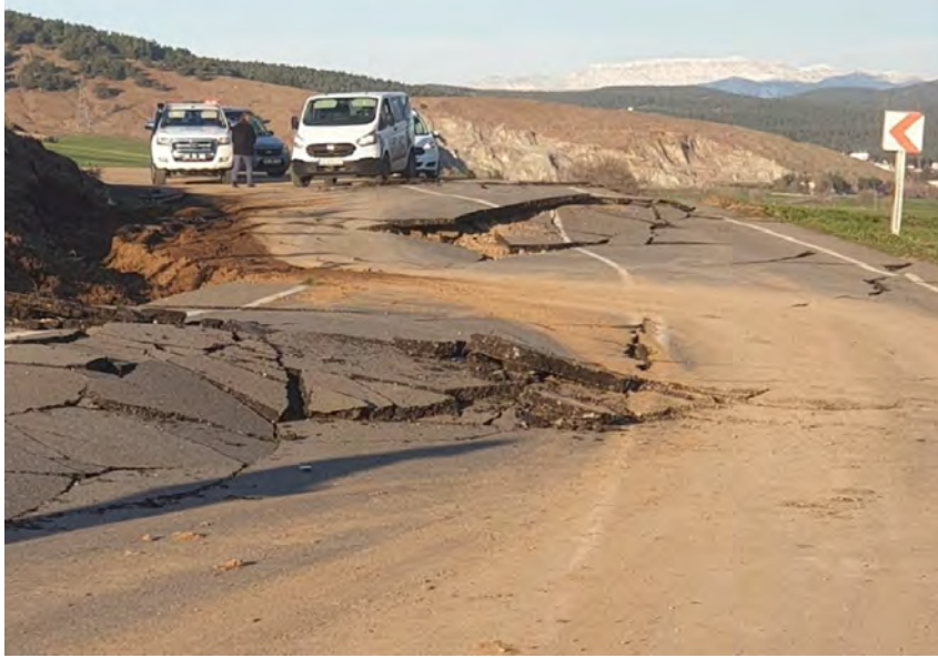
Figure 21: Road damage in Tevekkeli, Tevekkeli Village Road, 46090. (Source: Twitter Zeliş; https://twitter.com/Panthalassa_Z/status/1623237597752352769 )
