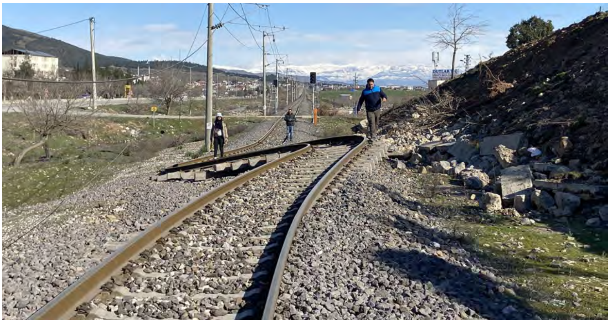
Figure 24: Surface displacement in Şekeroba highlighted by rail displacement (Source: Twitter Cengiz Zabcı https://twitter.com/CengizZabcı/status/1623236454926229504/photo/1 )
