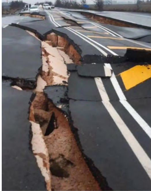
Figure 23: Road in Hatay, Turkey completely split open. (Source Video: Video https://twitter.com/porcumali/status/1622594257176469506 )
