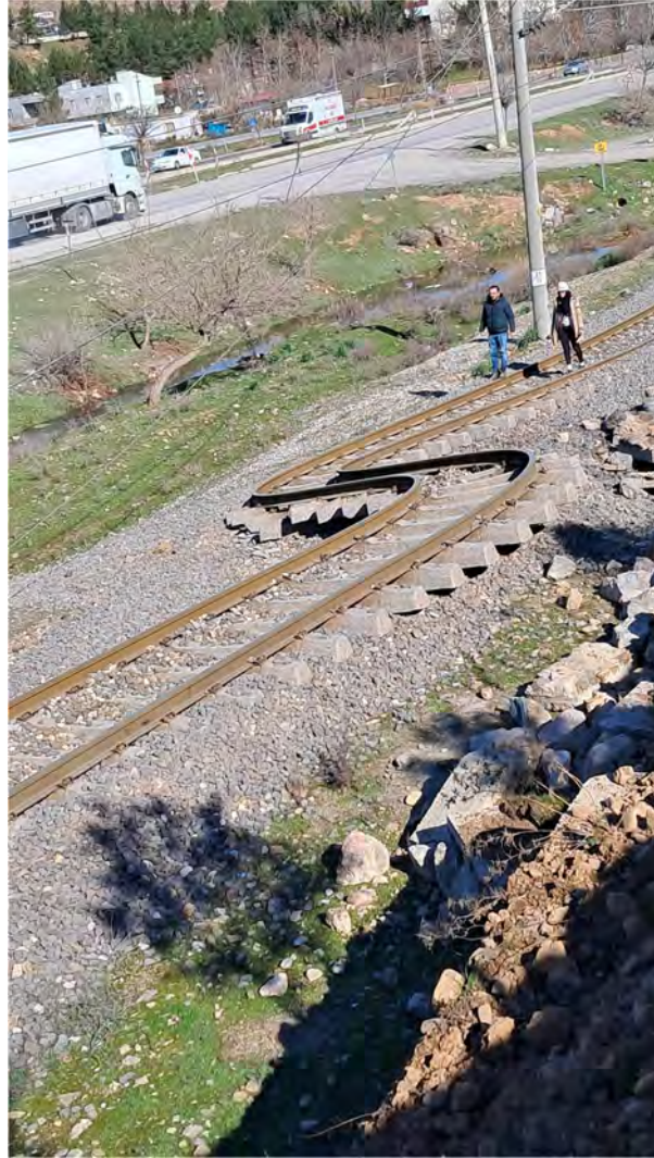
Figure 25: Surface displacement in Şekeroba highlighted by rail displacement (Source: @akyuz24 on Twitter)
